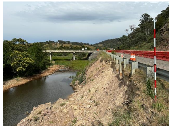
Plate 4: Southern verge with view of bridge intersection with heavy erosion along Mulwaree River (West)
