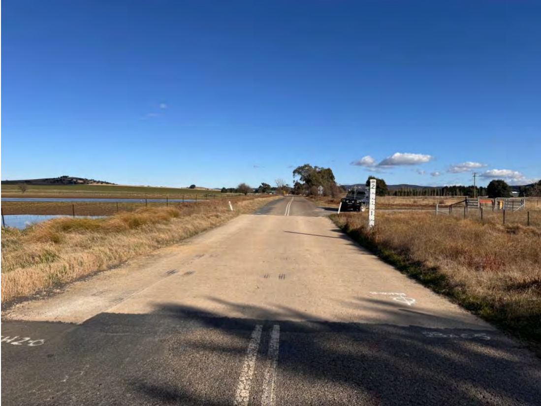
Photo 3; Causeway at Ch1864 requiring replacement, facing west
