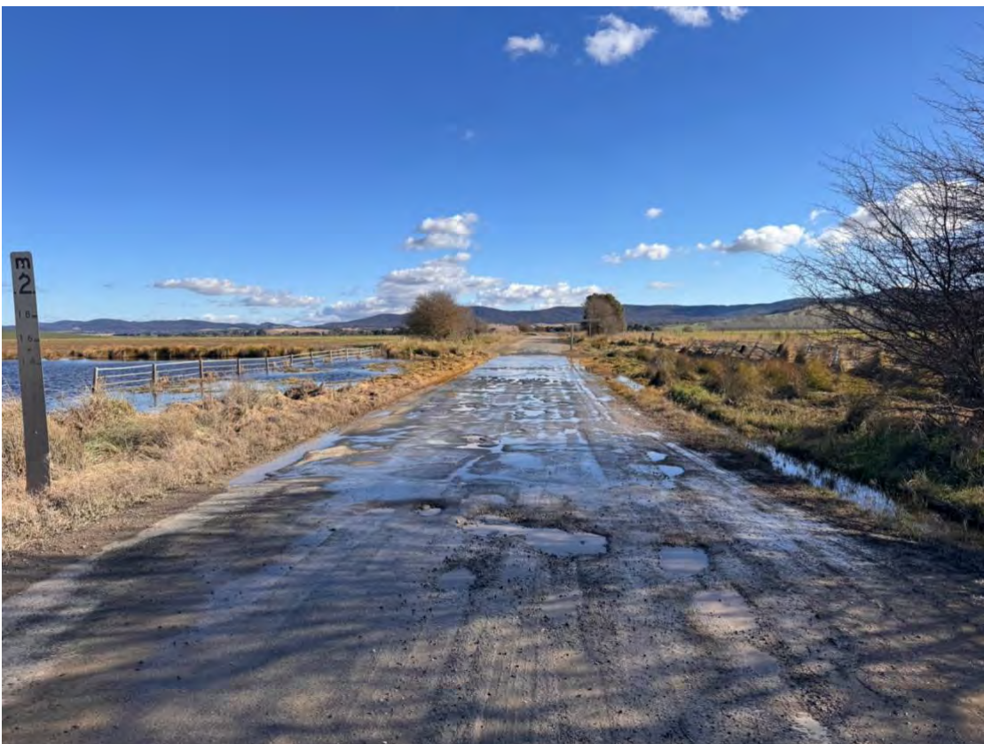
Photo 2; Saltpetre Creek causeway requiring replacement, facing west.
