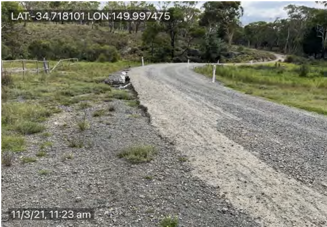
Causeway Erosion Repair works on Barbers Creek Rd - Before
