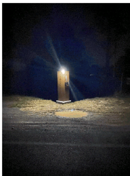
Avenue of Honour Signage Lights
