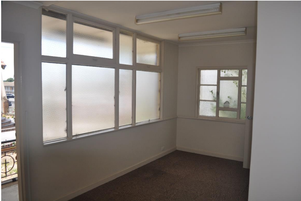
Internal view of the verandah, the windows will be removed, and the internal lining returned to the original face brick
