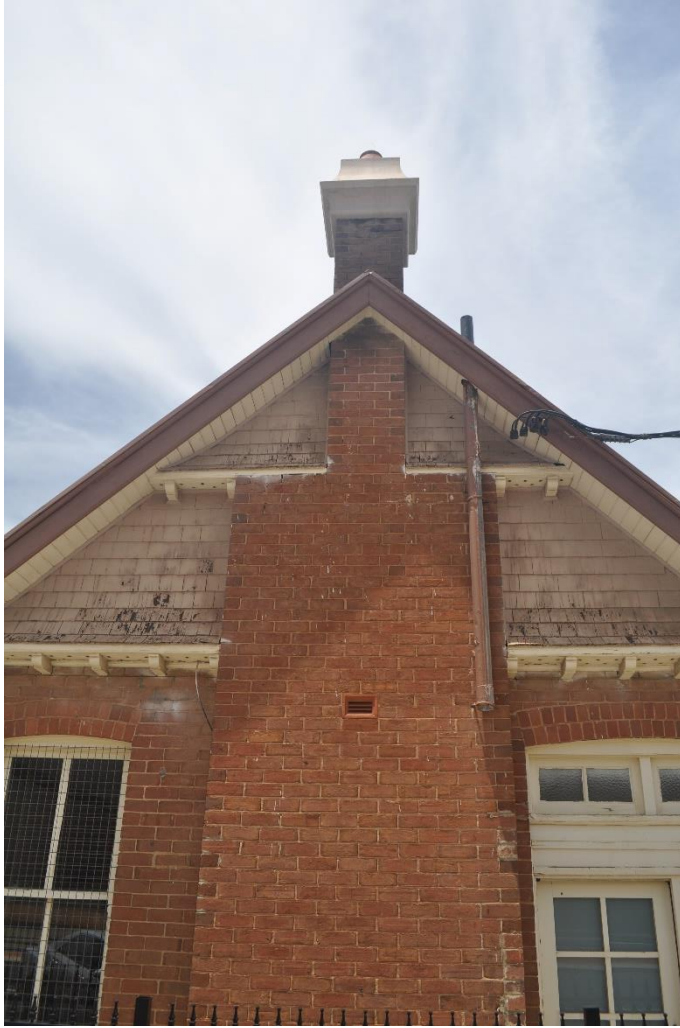
Detail of the Western chimney and gable end. The timber work will all be restored.
