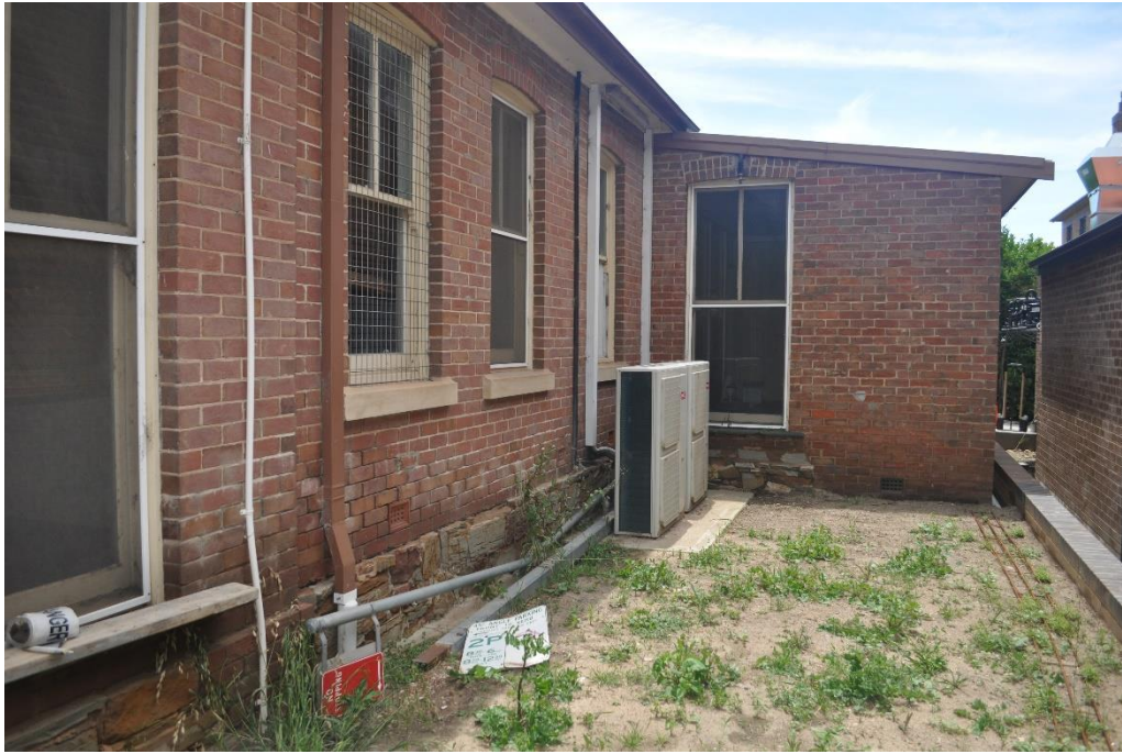
Detail of the eastern façade, note the damage from the downpipe leaking,
