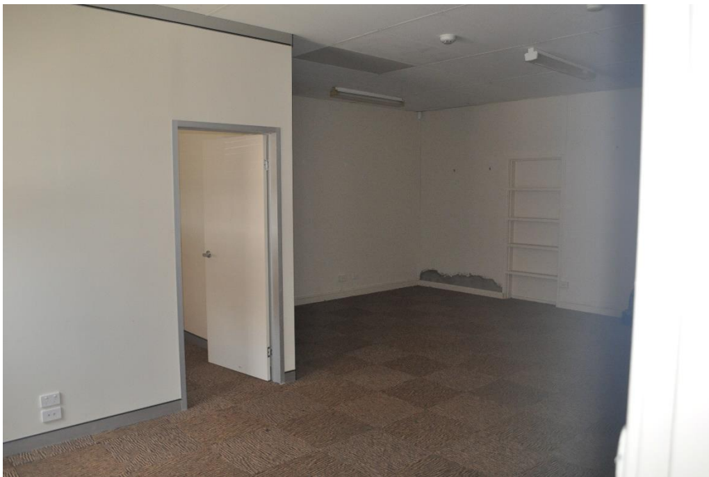
General view of the openplan office area. The existing partitioning will be removed as will the suspended ceiling system.
