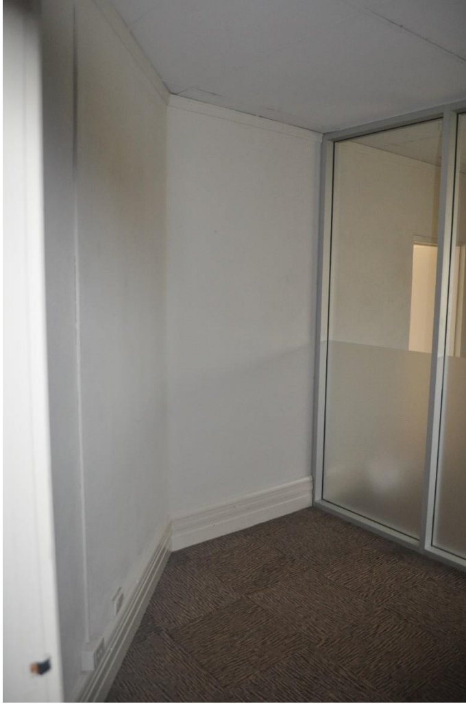
View of partitioned front room. This partition will be removed. Skirtings are original. The ceiling will be replaced.
