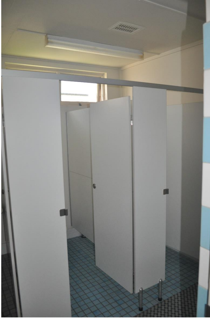
View to the refurbished male toilet with accessible facility (non compliant)
