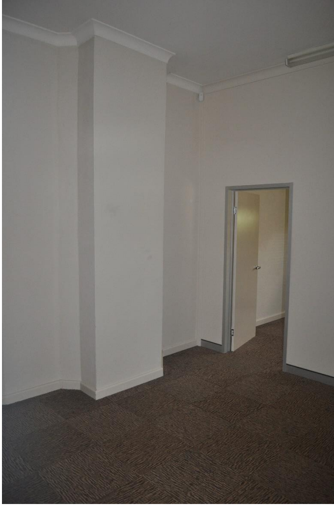
View of the entry to the South West front room (closest to the roundabout), this non original partition will be removed
