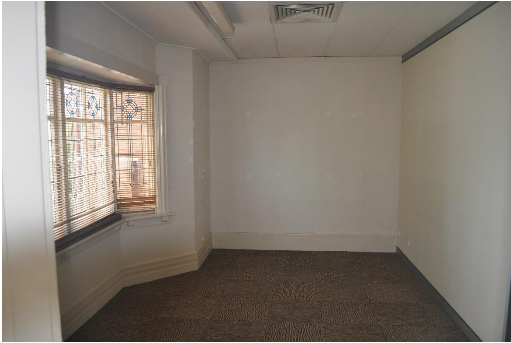
Internal view of the main front room. The original window remains intact and will be refurbished. The partition to the right of frame will be removed. Note also the non-original ceiling. This will be replaced
