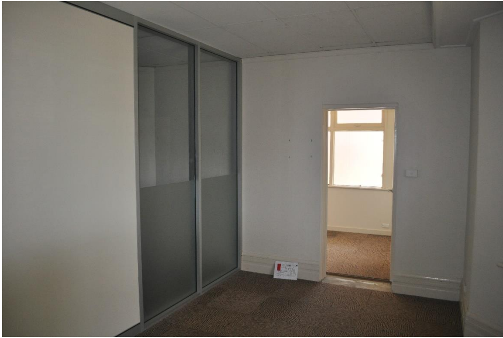
View of the same room detailing the glazed section of the partition to be removed. The veranda is visible beyond. The doorway will be bricked up as part of the proposed renovation. The door was not original.
