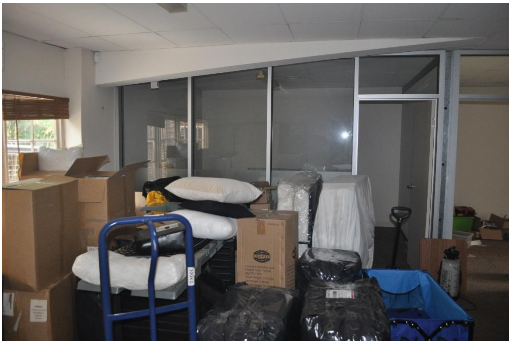
View to the North of the same area note the roof structure
