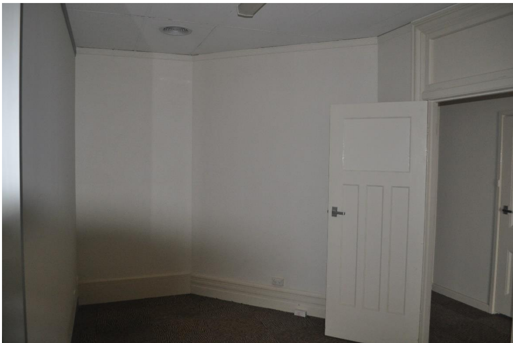
View back to the entry from the main corridor. This will become the main waiting area.
