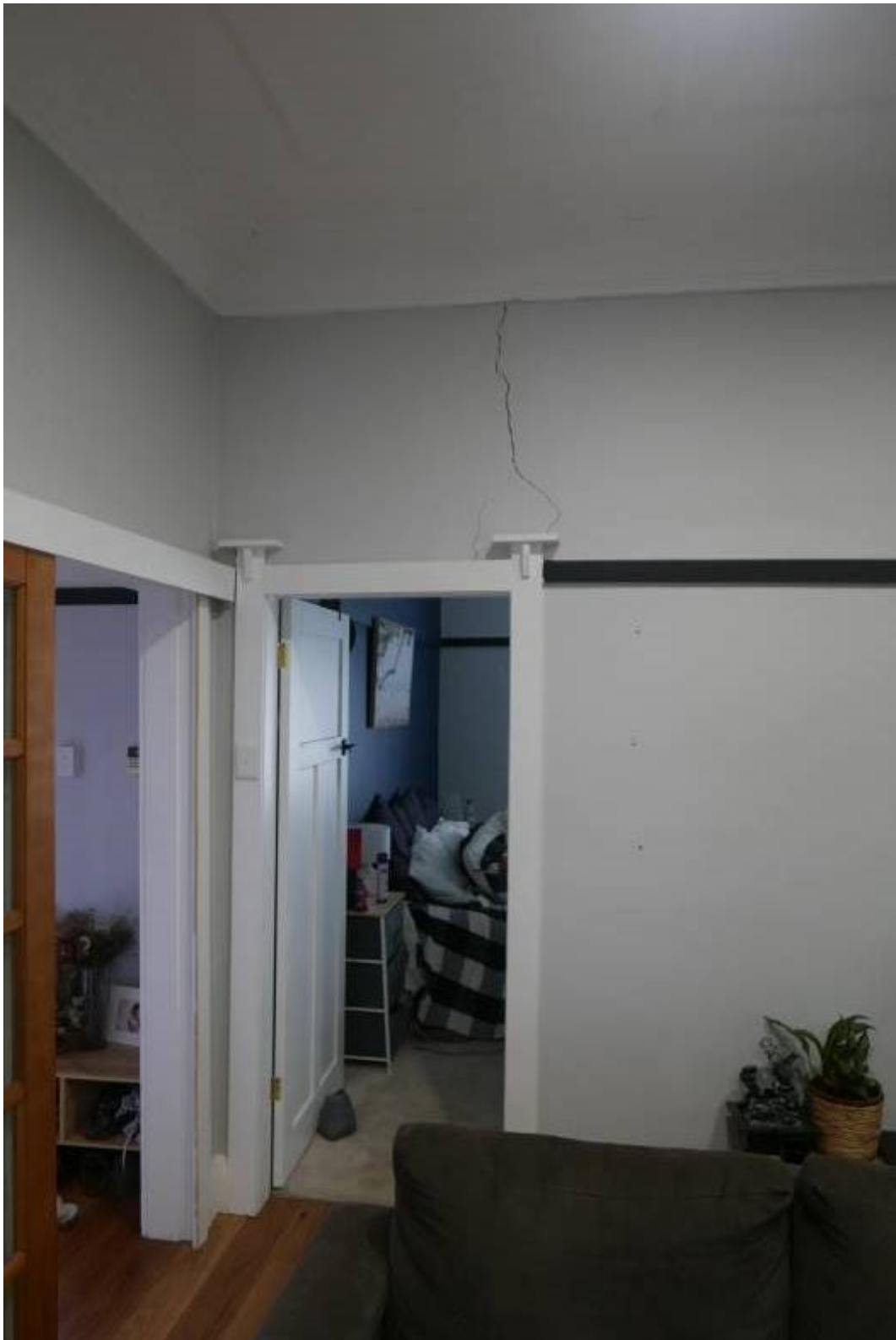
Photo 2 – Crack in wall in living room.
