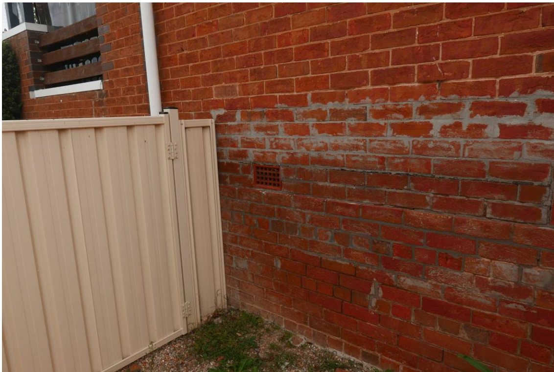
Photo 14 – Typical condition of external brickwork. Note the common bond with full headers every 4 th course.
