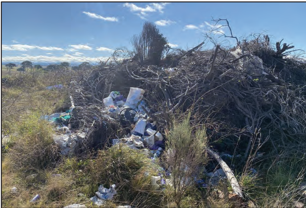
Photo 11: View of waste material on ground in fill platform area
